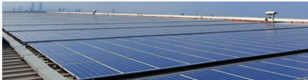
Roof-Mounted Photovoltaic Power Station
